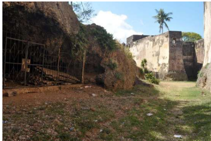
Figure 18: Coral cave in the ditch outside south western side of Fort Jesus. Notice a pile of asbestos which is harmful to human health. The asbestos should be disposed of by licensed handler under supervision of National Environment Management Authority. Photo by Stephen Okoko.
