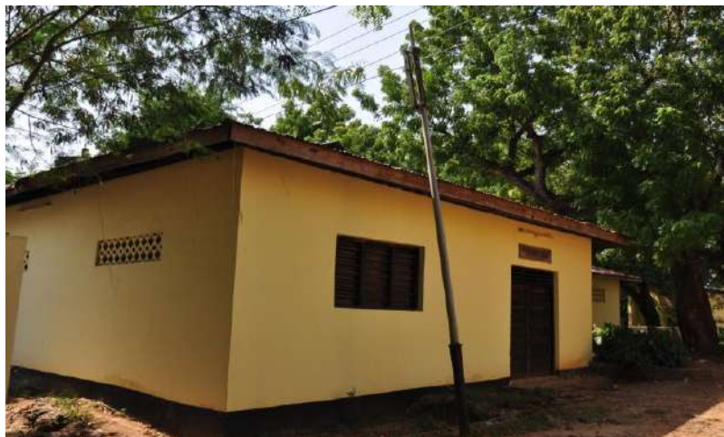
Figure 4: Outside the archaeological storage building. An insulated electricity main power lines slightly above the roof. Photo by Stephen Okoko.
