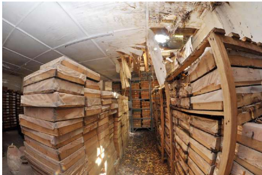
Figure 10: Inside Archaeological Storage Room. Notice the derelict condition of the roof structure and ceiling of the building. Revamp the roof and ceiling and replace wooden drawers and shelves with metallic and plastic ones. Photo by Stephen Okoko.
