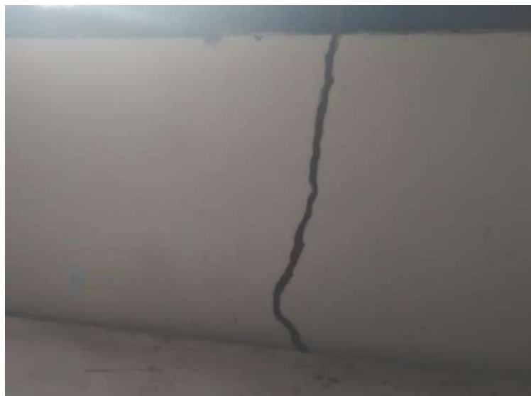
Figure 14: Inside Archaeological Storage Room. Notice the termite infestation on the wall which threatens the preservation of the collection in the storage room. Regular pest control measures required. Photo by George Ghandi.
