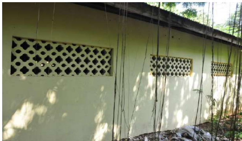
Figure 6: Outside the archaeological storage building. The poorly designed windows impede ventilation and control of dust inside the storage room. The vegetation growth provides ideal environment for mosquito breeding. Photo by Stephen Okoko.
