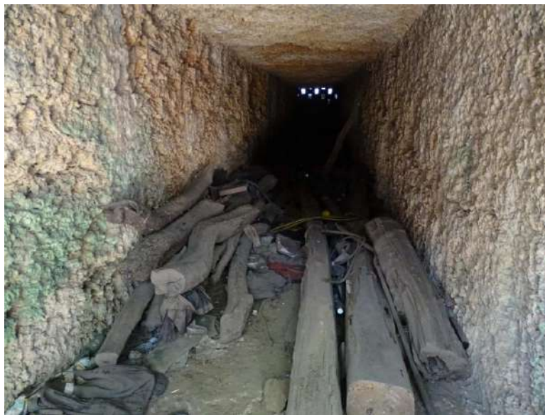
Figure 20: Military tunnel cut through coral formation outside Fort Jesus. It can be cleaned and presented to public as part of tour trail around Fort Jesus. Photo by Stephen Okoko.
