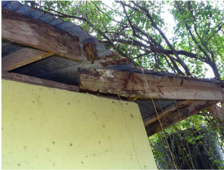
Figure 5: Outside the archaeological storage building. Notice broken fascia board at the northwest the corner. Rehabilitate entire roof structure of the storage building. Photo by Stephen Okoko.
