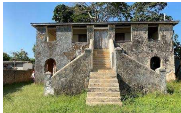
Plate 9: Surface blackening, Colonial headquarters
