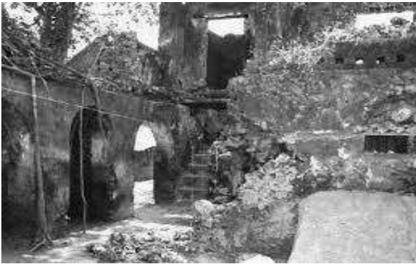
Plate 12: Collapsed historic building
