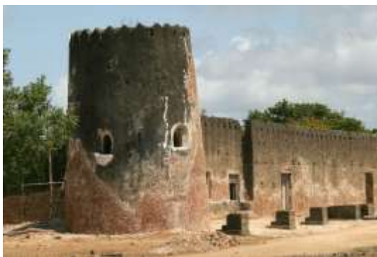
Plate 2: Surface blackening, Siyu Fort (Source: Njiiri et al., 2025a)
