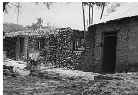
Plate 10: Damaged wattle-daub structures (Source: Authors, 2026)
